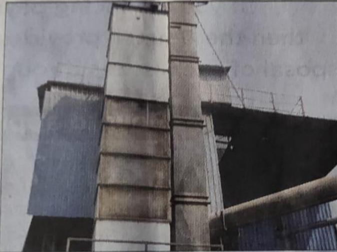
The device will capture carbon dioxide and sulphur dioxide and reduce temperature of waste gases. FILE PHOTO
